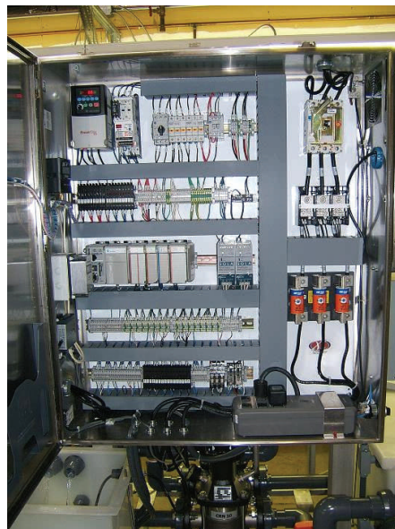
Advanced control systems can operate many parts of the modern processing plant.
